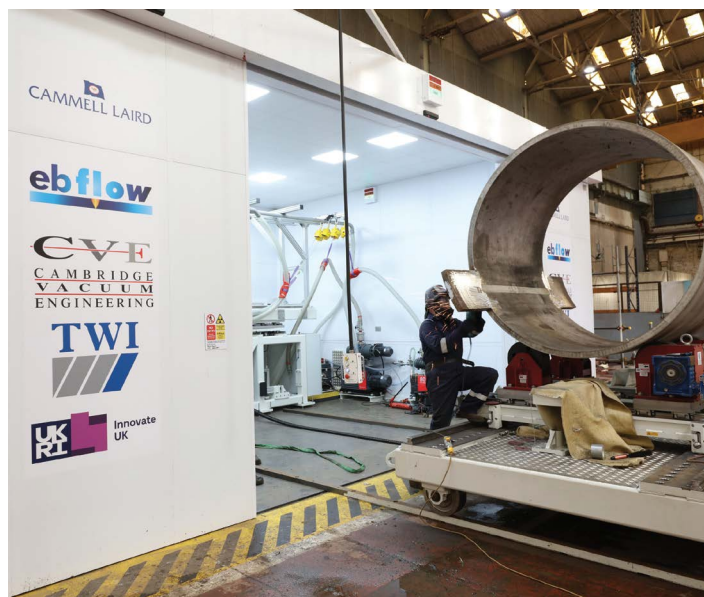
Figure 3: Ebflow system installed in Cammell Laird shipyard for fabrication of demonstration nuclear pressure vessel in support of the EBManpower project. © published courtesy of the EBManPower Project.
