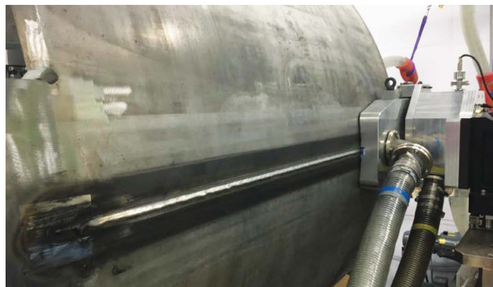
Figure 2: Fully penetrating linear weld in 60mm thickness 304H grade austenitic stainless steel – completed in 8 minutes of welding time. © published courtesy of the EBManPower Project.
